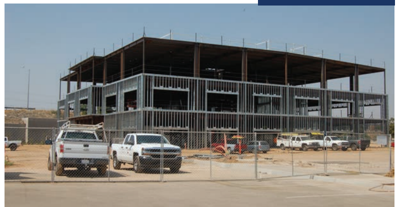
PHOTO BY FRANK LOPEZ | This March photo shows the progress of construction on a three-story office building in Fresno on Nees Avenue just south of Friant Road.
